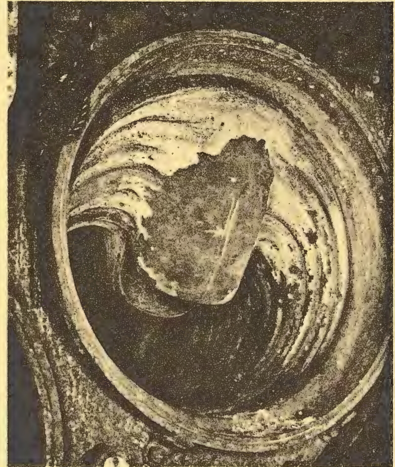
FIG. 39.—FAILURE OF A SCOTCH BOILER FURNACE
